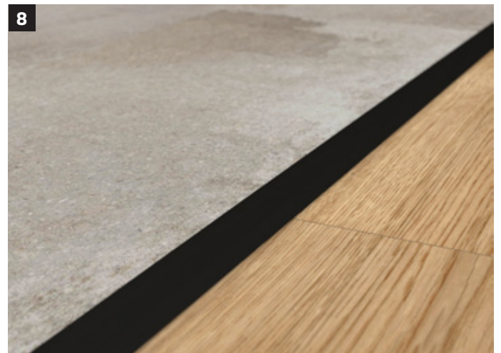
The transition profile is installed. After a brief inspection, the next section can be assembled.
